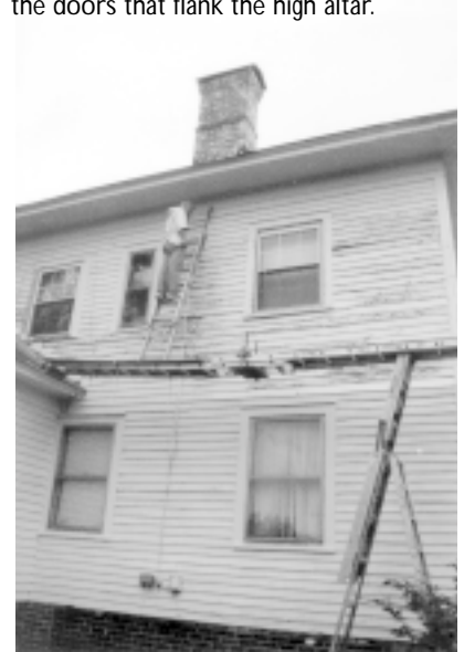
A view of the clapboard restoration in progress. Note closely the interesting scaffolding arrangement, complete with C-clamps!
