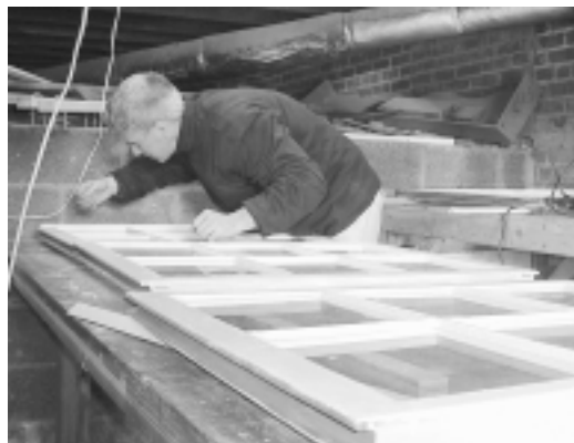
In the basement garage, the restored windows takes shape, complete with new glass panes and caulking.
