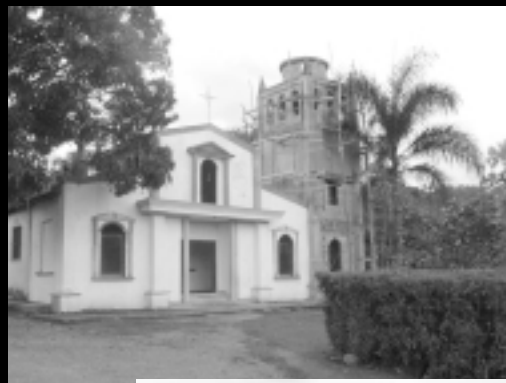
Construction of the bell tower for a new chapel in Santo Domingo continues.
