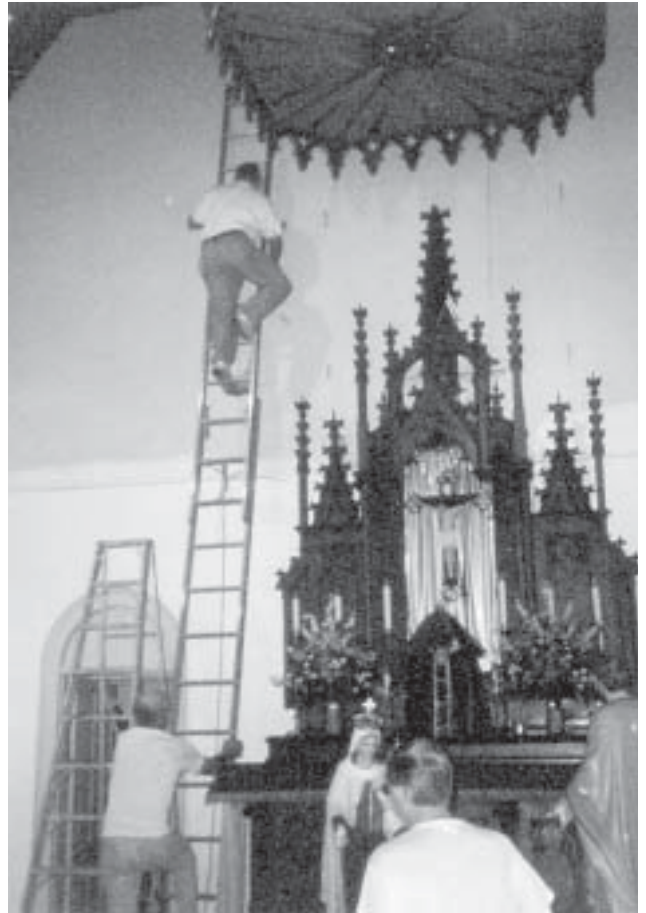
New wallboard lines the front wall behind the altar that was installed years ago by former pastor (now in Arcadia, CA), Fr. Charles Ward. Here, parish painters are getting the hard spots.
