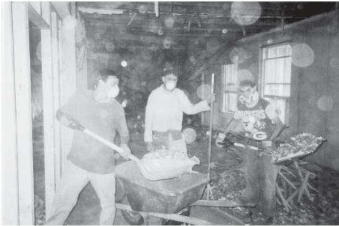
After the fun job of tearing down plaster lath walls and ceilings comes the seemingly never-ending and extremely dusty job of cleaning up the mess! The dust is so thick in fact, that it has even spotted the camera lens in this shot.
