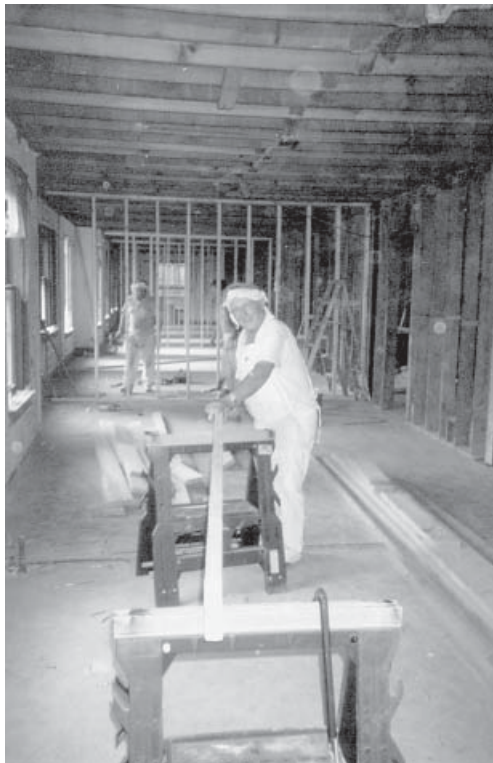
Here we can see the new framing for partitioning rooms being cut and put into place. Next the wiring, plumbing and dry wall will need to be installed.
