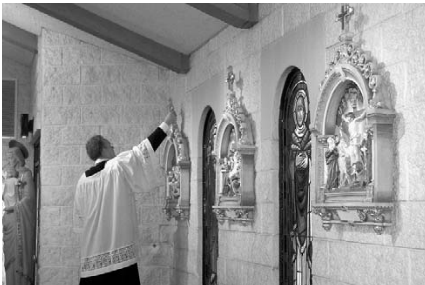
Fr. Ward installs the wooden cross on the Fourteenth Station, “Christ is laid in the Sepulchre”. Though the decorative part of the Stations may be made of any type of noble material, every Station must have a wooden cross somehow incorporated in order to remind those who make the stations of the “ Lignum Crucis ”.
