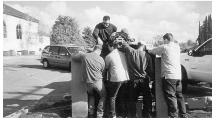
Several men of the parish carefully wrestle the solid piece of granite into grooves made on the inside walls of the pedestals.
