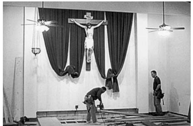
A shot of the beginning stages of the remodeling process. The single step has been removed in preparation for the addition of the new three stepped predella.
