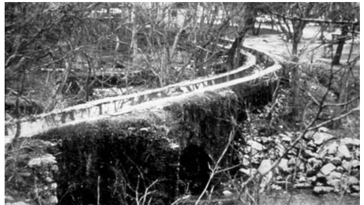
A partial view of the still-working stone aqueduct situated not far from the Mission San Jose. The Spanish missionaries built an interconnecting system of acequias (a network of gravity-flow ditches whose use originated in Moorish Spain), aqueduct and 5 dams covering 15 miles to provide water for 3,500 acres of farm land.
