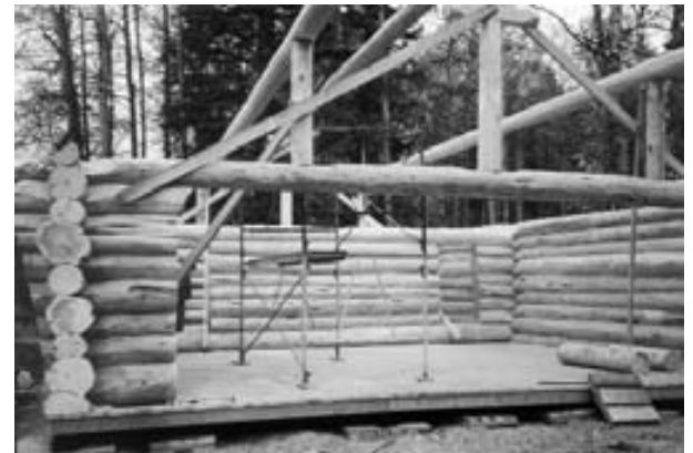
The new log chapel in honor of Saint Joseph being erected. The floor was laid by the boys of the parish, who camped out and spent two days laying the pallets (seen below the floor), which in turn support massive horizontal logs that support the floor framework. Afterwards, the boys remarked that "it was the best fun we ever had!"
