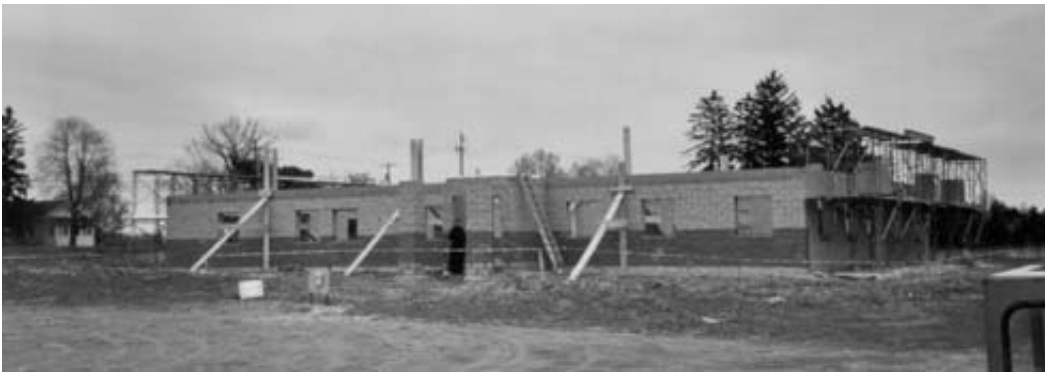
Father Libietis stands beside the walls of the building in construction. The photo is taken looking towards the main road.
