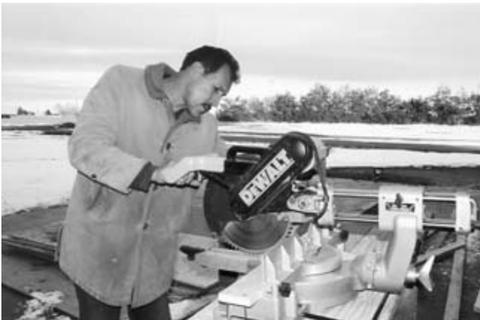
Snow on the ground does not prevent Holy Name member Ramon Gasca from mitering a section of trim for the church.
