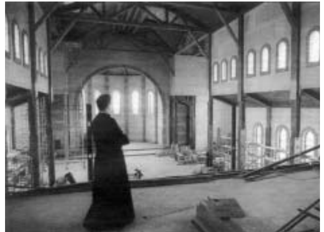
Father Joseph Pfeiffer, the pastor, gazes at the progress of construction from the choir loft of St. Isidore's.
