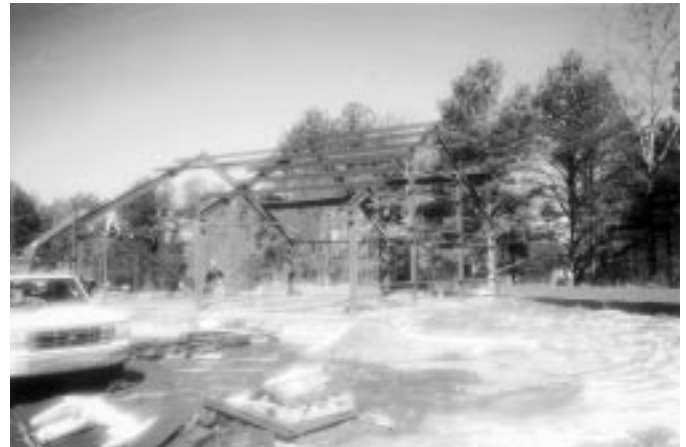
The erection of the simple rectangular steel frame building on a concrete slab.
