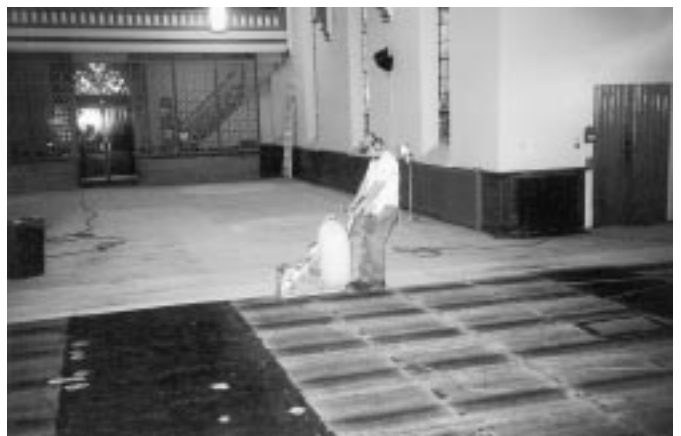
The sanding of the floor, starting from the back and working towards the front of the church.
