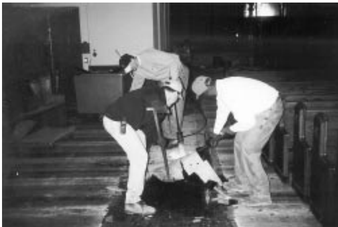
Workers had to use a blow torch to remove the glue and old floor coverings under the carpet runners.
