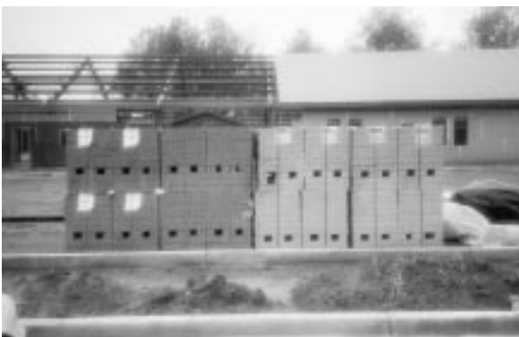
Loads of bricks for the exterior facing arrive on the parking lot.
