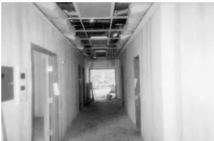
A view up the main hallway, leading to the chapel at the far end. Catechism rooms, a kitchen, and a priest's apartment are off this main hallway.
