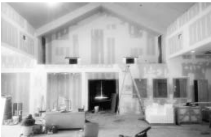
Looking back in the church towards the choir loft, still in construction.
