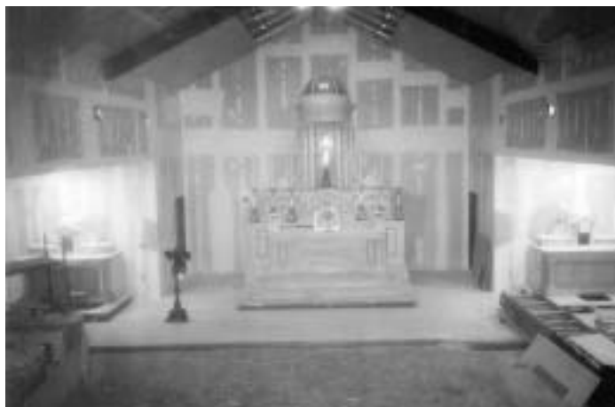
A view of the sanctuary of St. Michael's still in construction, but with the three marble altars already installed.
