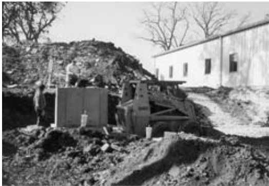
Digging out an underground water storage area to slow down the draining of storm water from the site.
