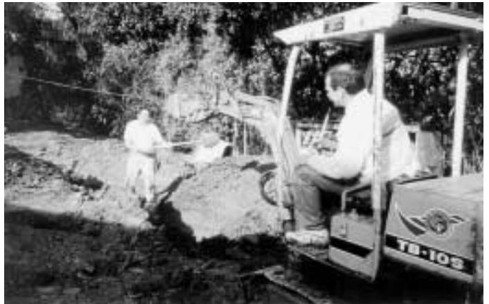
Replacing an old waterline on the northeast side of the retreat house.
