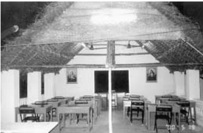
The study hall was constructed on the veranda, increasing our living space considerably!!
