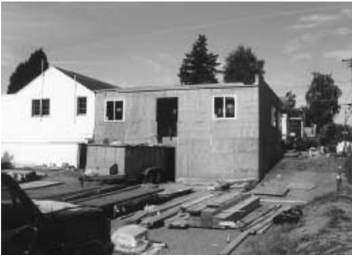
An uphill view of the construction in progress, taken from the parking lot below the parish hall.
