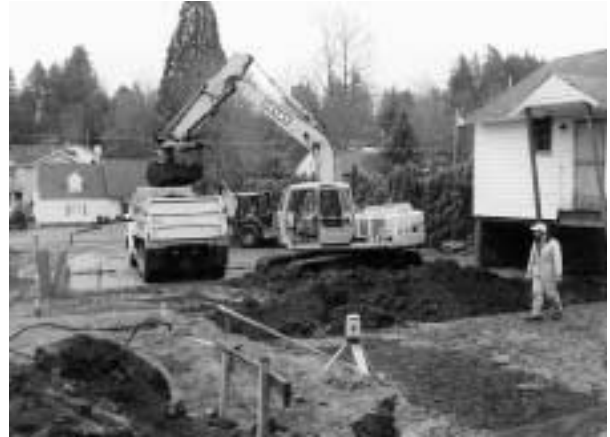
Excavation for the new extension begins, in the quadrangle that used to separate the parish hall and the chapel.
