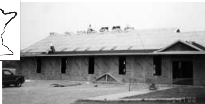
A close-up of the addition, as men and Academy students begin the roofing work on their new building.
